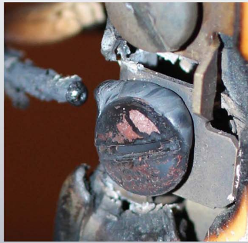
Severed Conductor (Welded w/Curved Striations)
