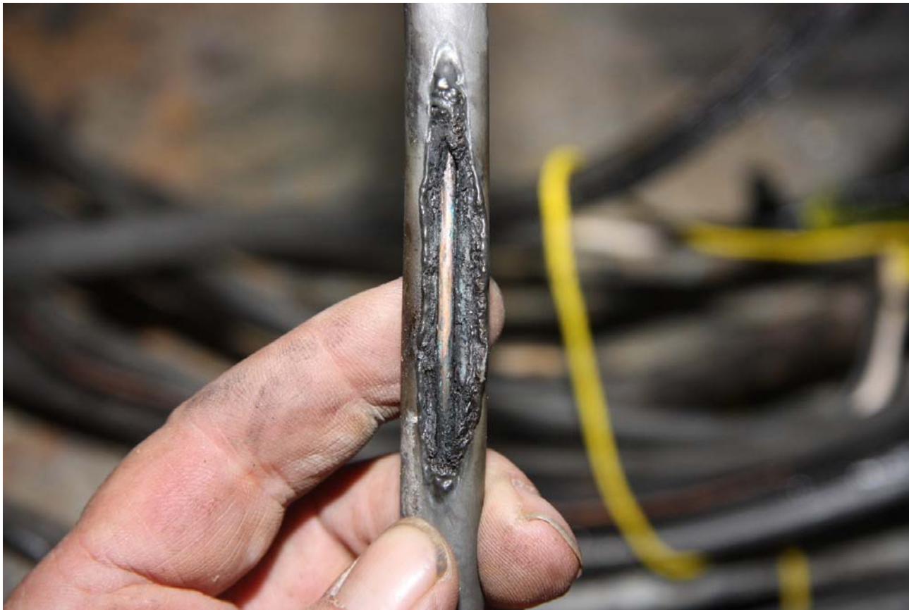
F08-049: Localized Melting at the Grounding Conductor
